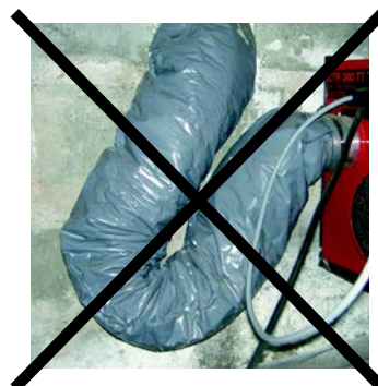
Feil montering, sterk bøy
